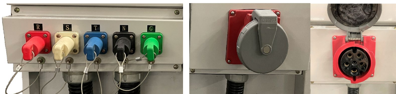
Figure 3.6- Additional Power Supply
