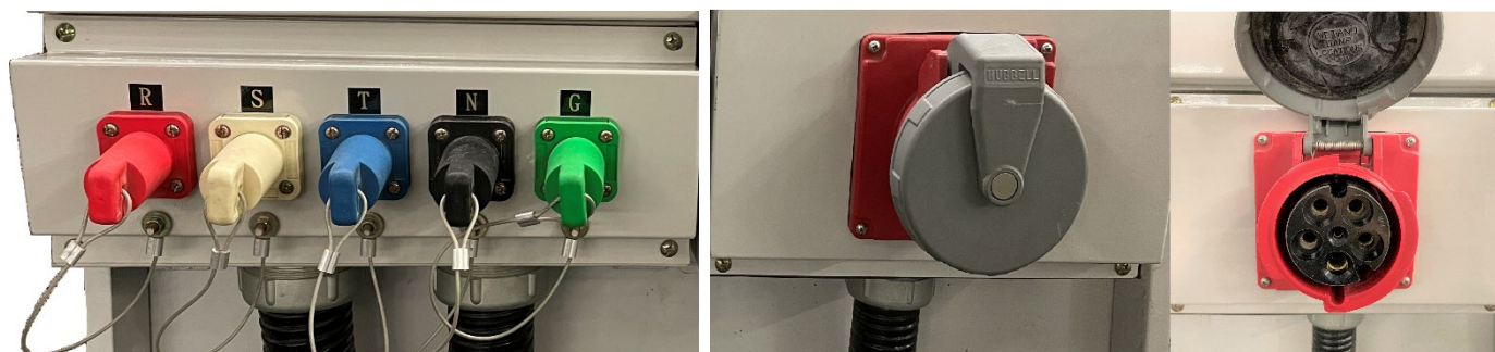
Figure 3.6- Additional Power Supply-Camlock, CEE125
